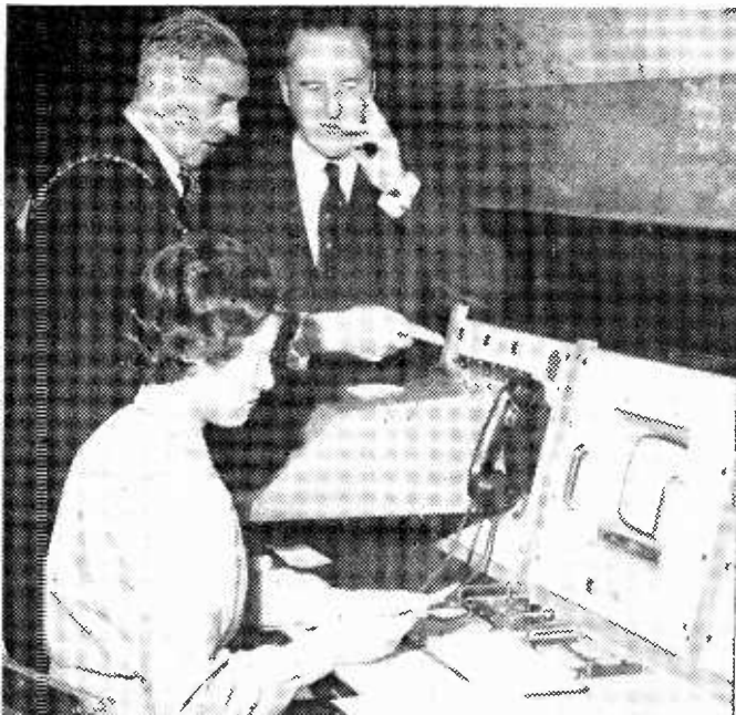
Branches of the Westminster Bank in Manchester have been connected with each other by means of a closed-circuit TV system. Here the Lord Mayor of Manchester (Ald. H. Quinn), watches the start of the televising of accounts from Branch to Branch.
